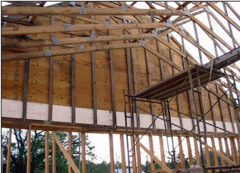
Figure 7-14. Improperly braced gable walls. The ceiling diaphragm (i.e., the bottom chords of the scissor truss) is located several feet above the top of the end wall top plate and no wall-to-truss bracing is provided. (Source: FEMA 549)
