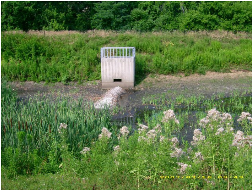
Concrete riser with horizontal dewatering device
