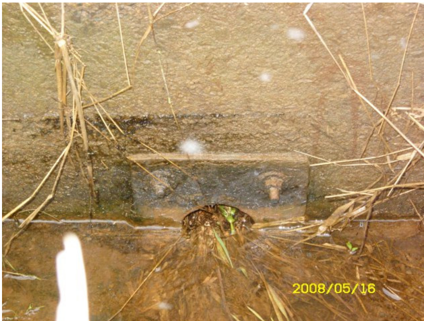
Clogged low flow orifice
